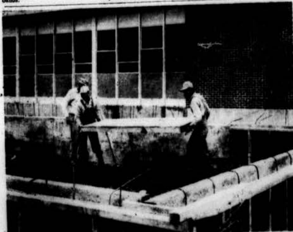
STUDENT UNION EXPANSION — Employees of the O. D. Fritz Construction Company of Vinita are shown here working on the expansion of the Bruce G. Carter Student Union Building. This is only one phase of building and progress on NEO's campus. Photo by Mike Grimes
