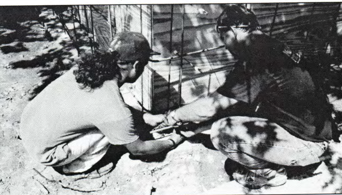
Jose Salazar (left) and John Turner, members of the college physical plant, prepare a form for concrete work around one of the many trees on campus.
