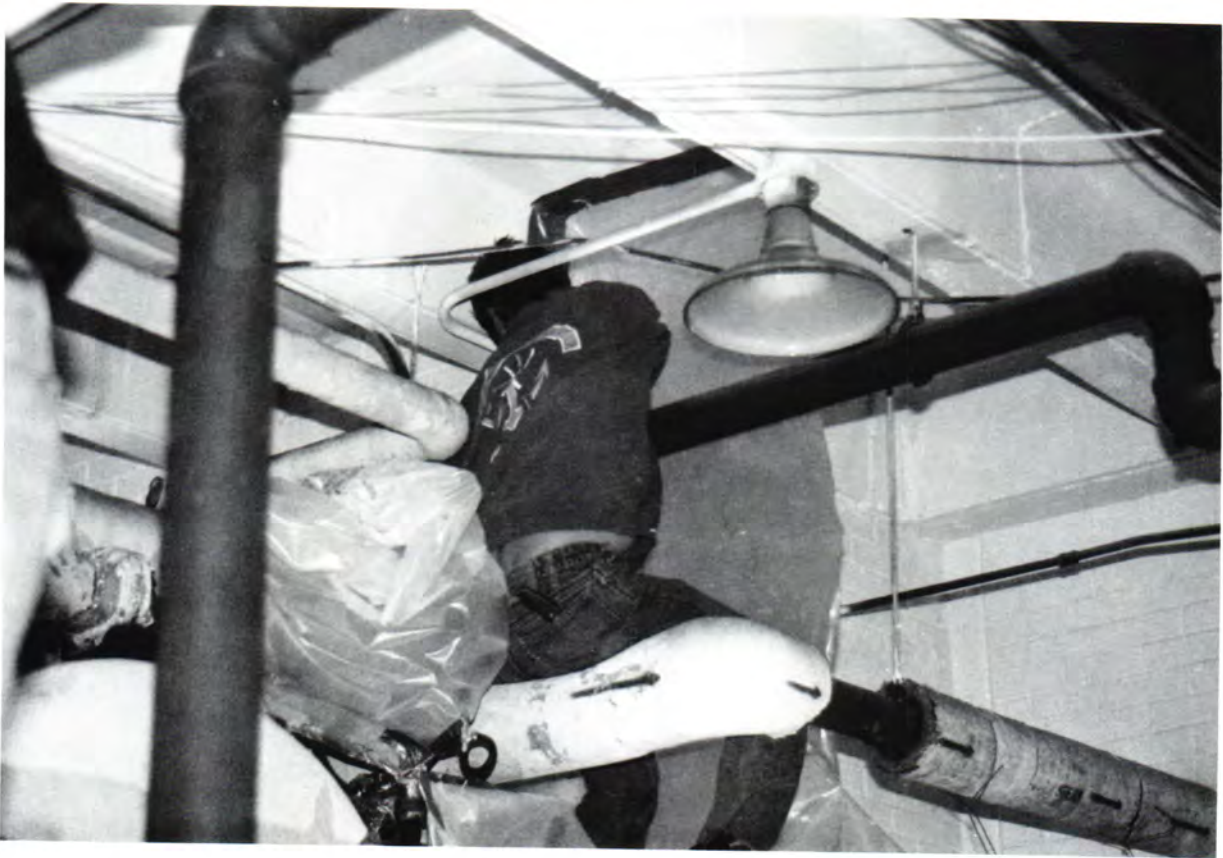
A worker from Crossland Construction sits on a pipe as he works to remove asbestos from the Dyer Hall plumbing system.
