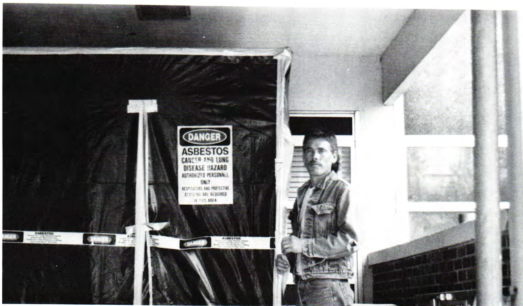
Taking a break before returning to removing asbestos in Dyer Hall is Danny Frost of Crossland Construction.
