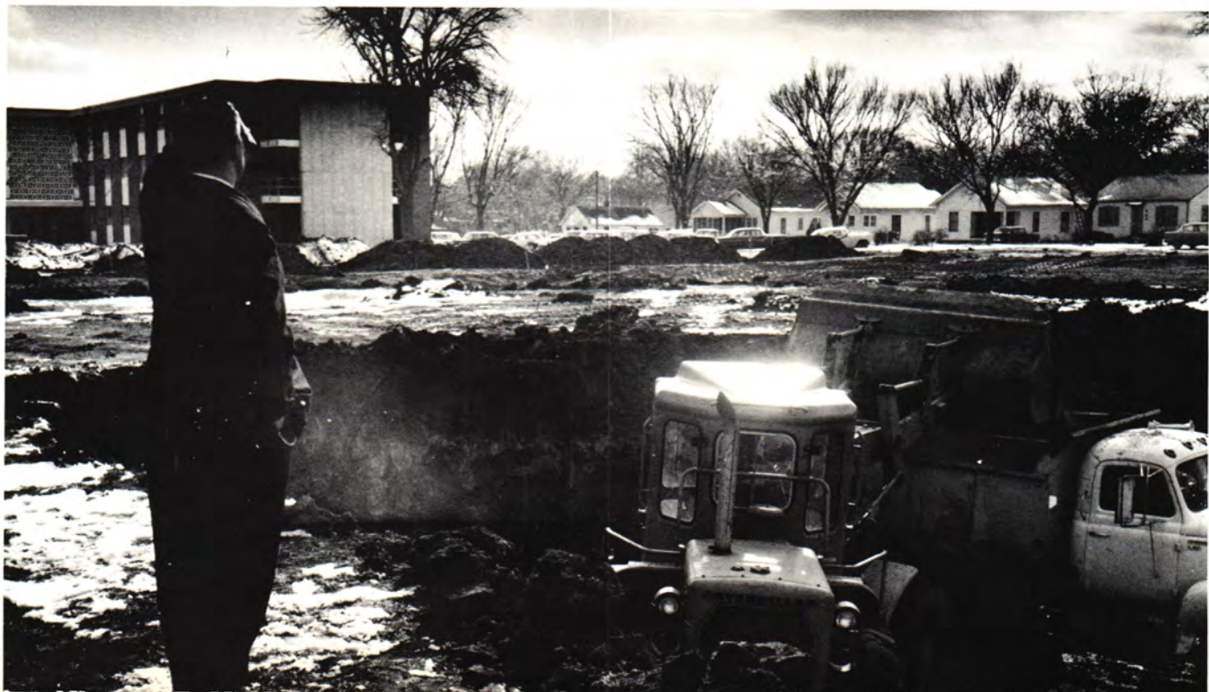
Dr. Bruce G. Carter, President of Northeastern Oklahoma A&M, views the beginning construction of the new administration-library building.
